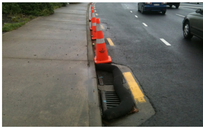
Installation of a silt sock to provide some protection to the catchpit
