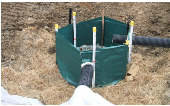
Good use of a silt fence installed to protect a new stormwater catchpit where impounded water will not create a flooding hazard
